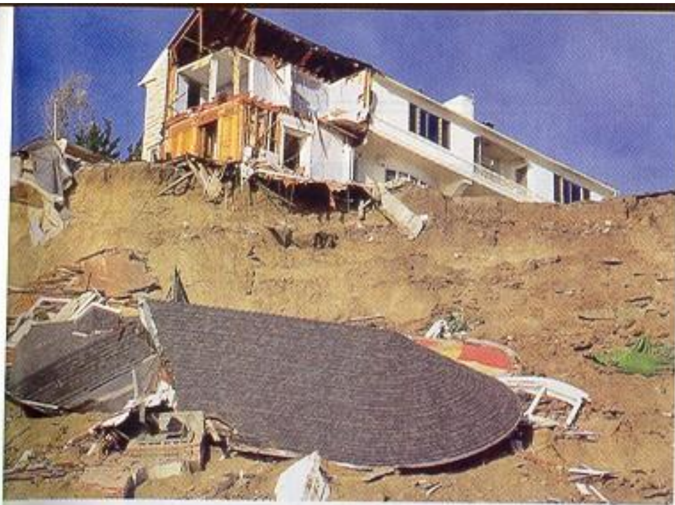
Figure 9.3 Various forms of mass wasting can be triggered by earthquakes. This home in Pacific Palisades, California, was destroyed by a landslide triggered by the January 1994 Northridge earthquake. In some cases, damages from earthquake-induced mass wasting are greater than damages caused directly by an earthquake's ground vibrations. (Photo by Chromo Sohm/The Stock Market)
